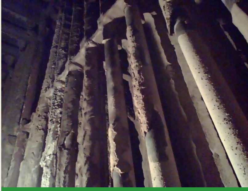
Ash Deposits On Super Heater Coils
